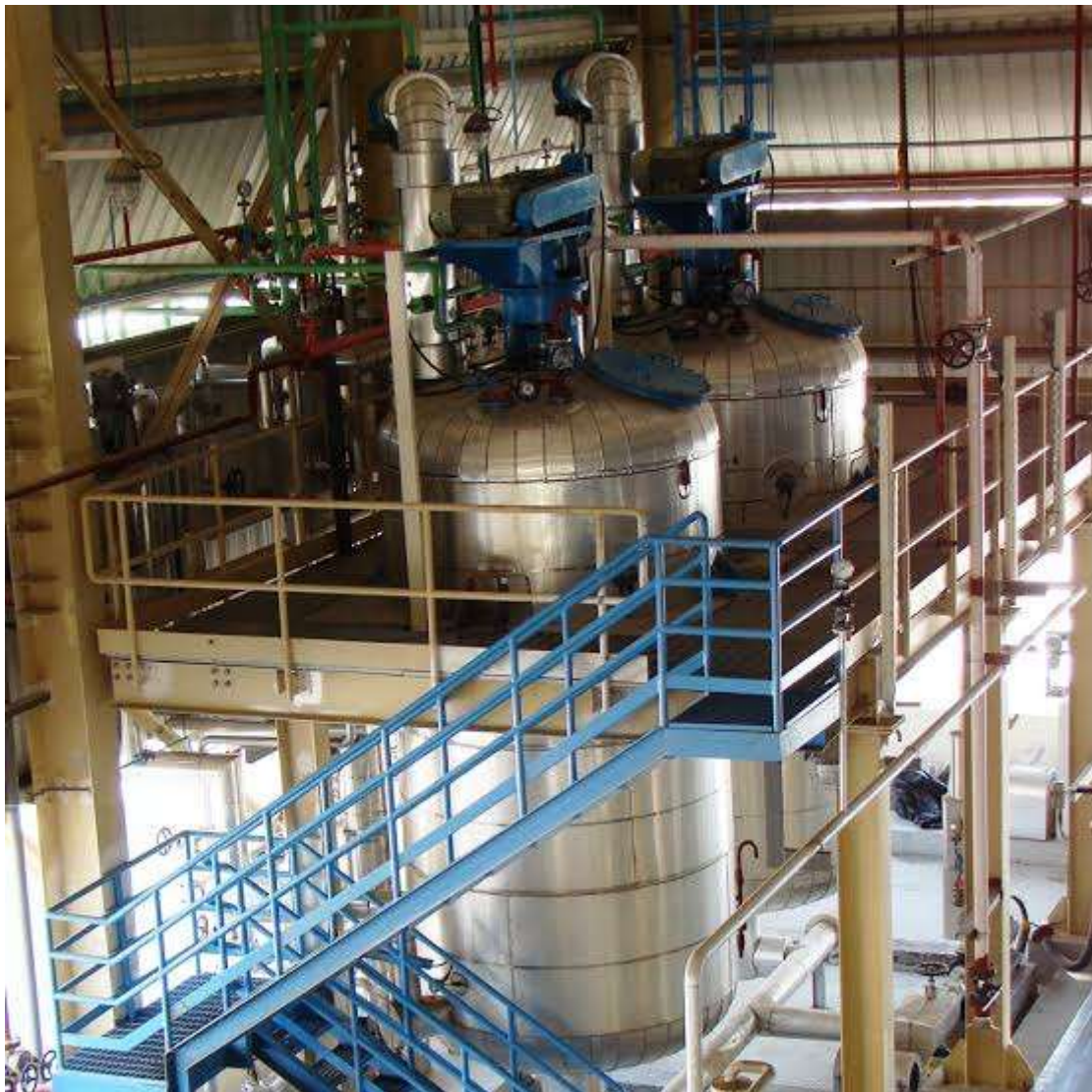
Figure 3: Automatic Blending plant
